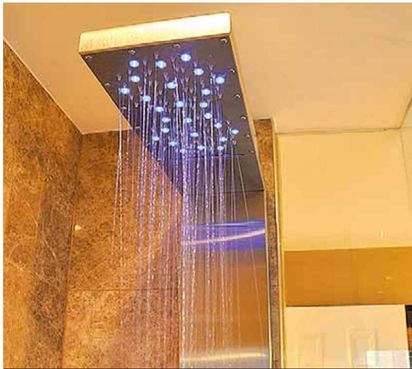
A shower column installation by RenoWOW in a Toronto condominium. SAM BENINATO
