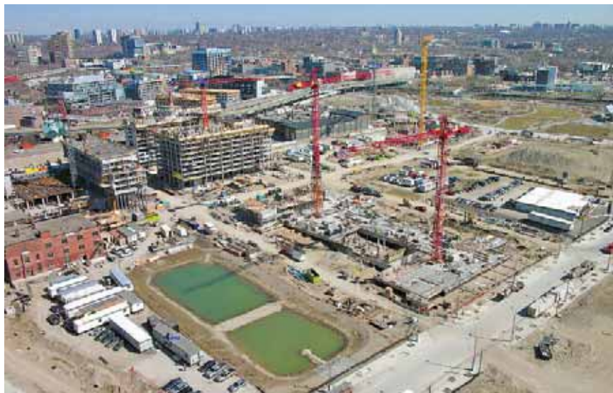
The West Don Lands site from the 26th floor of the still under construction Pure Spirits condo. DUNCAN MCALLISTER/FOR METRO
